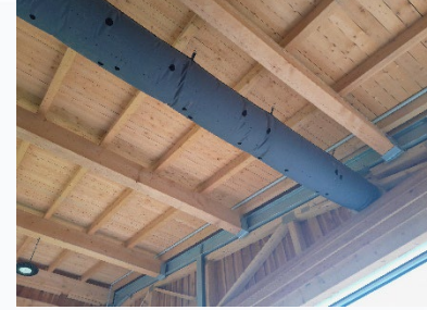
Tube ventilation system © I. Mösenbacher-Molterer
